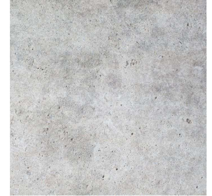
Fig . 33 – Example of Concrete colour to be used in scheme façade treatment
