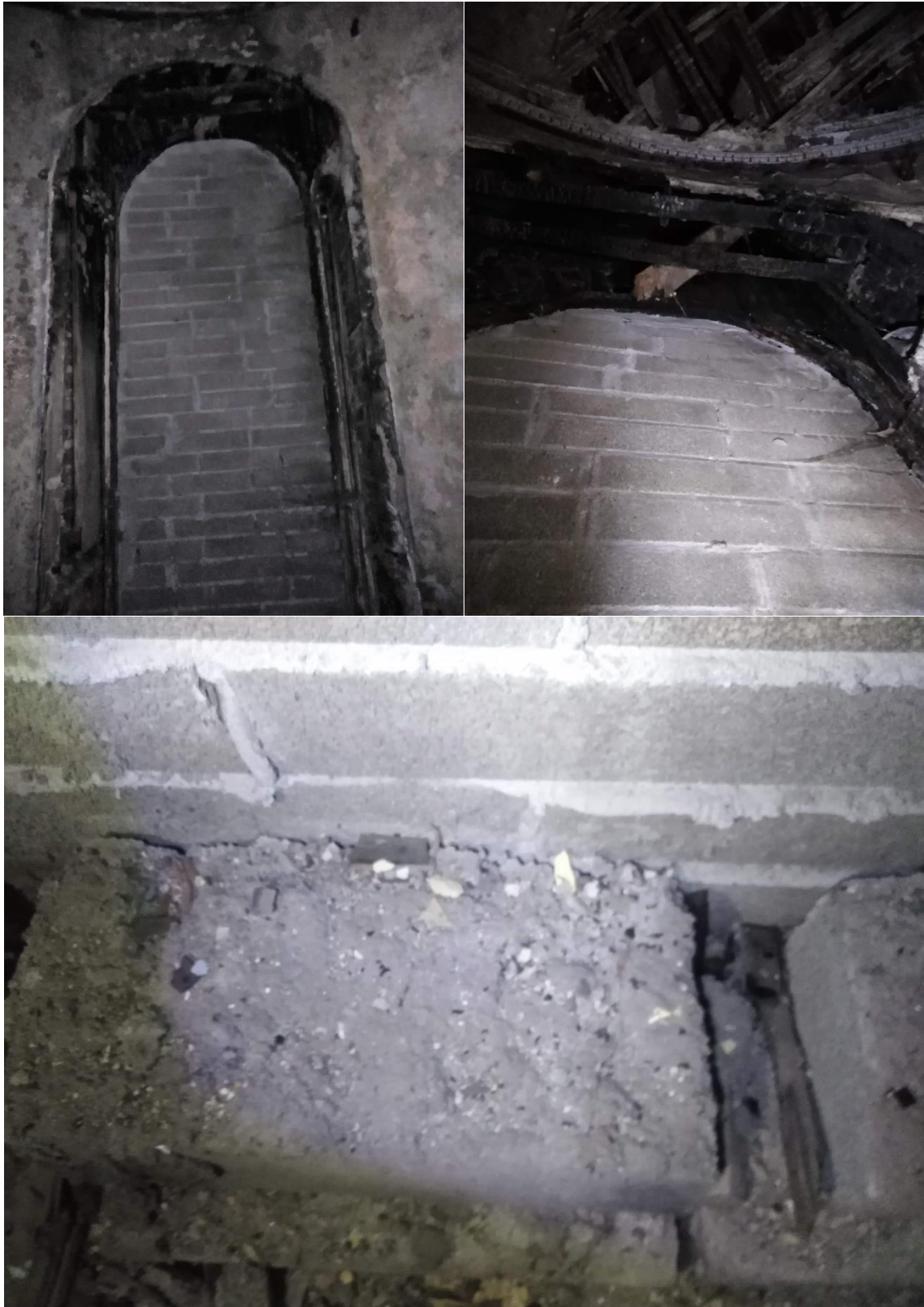
Bat droppings within a bricked-up doorway in the buildings in November 2019
