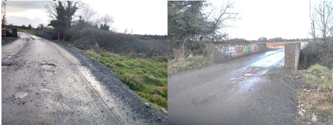
Bridge over the River Mayne, east of the site at the former Baldoyle racecourse area
