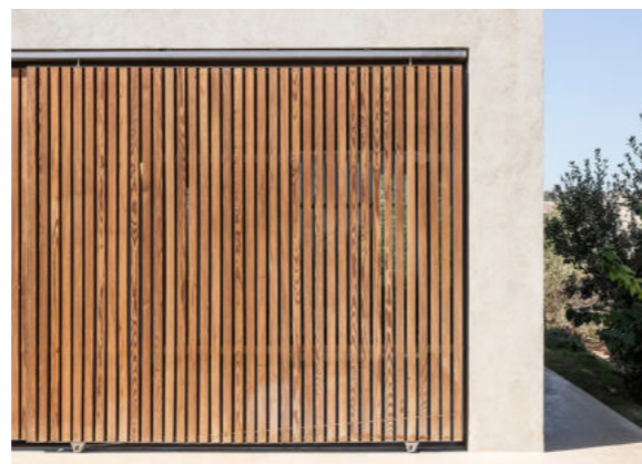
Timber slatted type doors to the communal areas on the north elevation
