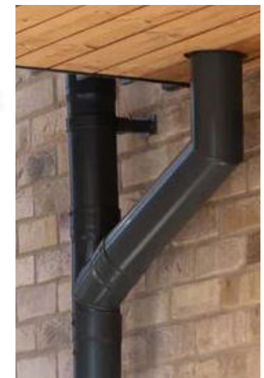
Drainage to the balcony
